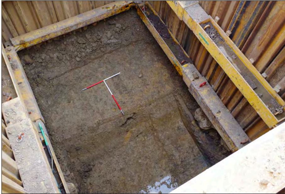
Plate 59: Trench 10 excavation conditions. Excavation has proceeded to the maximum extent of the arm of the mechanical excavator. The deposits in the base comprise moat bank deposits 10073, 10071 and 10072. Shot from north-west
