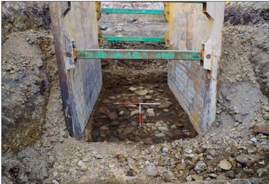
Plate 40: Working shot showing excavation conditions and relationship between medieval surface 5042 etc. (base of excavation) and bowling green wall 5010 (visible on left between green props). View from south
