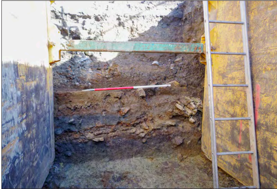
Plate 1: Working conditions in box shoring and west-facing section of trench 1 showing medieval layers and surfaces
